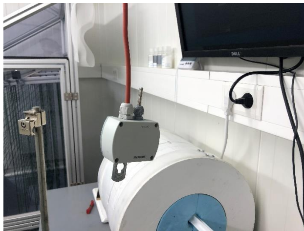
Figure 4 Temperature sensor installed above the test desk
